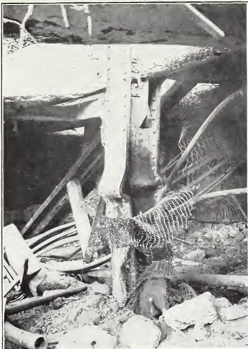
A. BUCKLING OF BASEMENT COLUMN DUE TO FAILURE OF PLASTERED METAL-LATH FIREPROOFING, RIALTO BUILDING, SAN FRANCISCO.
